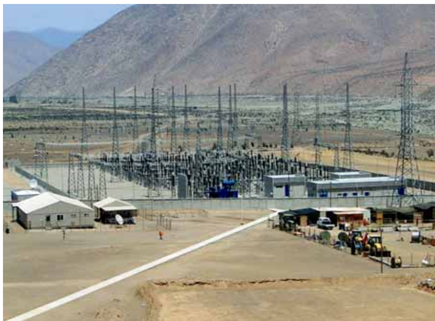
The primary substation at Punta Colorada, Chile connecting to the main power grid from which Pascua-Lama will obtain its electrical energy.
