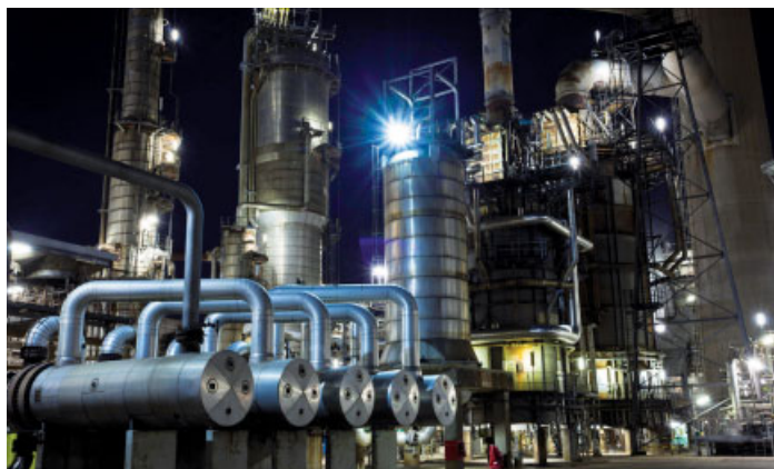
The storage tanks, pipes and towers at BP's Rotterdam refinery, which can run at least 70 different kinds of crude.
