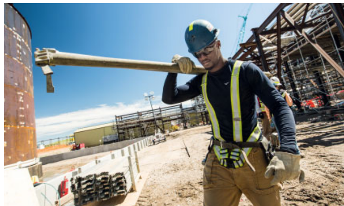
▲ Construction work on the Sunrise energy project, based in the Canadian oil sands of northern Alberta.
