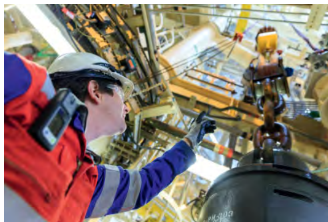
Above: On board Glen Lyon, our floating production storage and offloading vessel in the UK North Sea.
