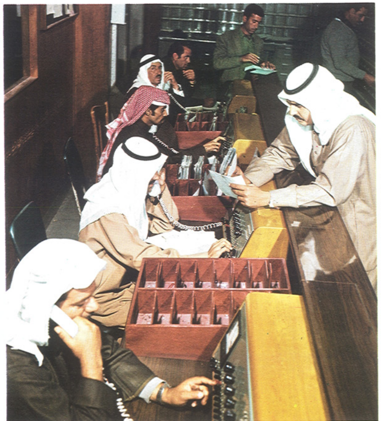
Testing subscriber lines in the automatic telephone exchange at Nuzha, Kuwait.
