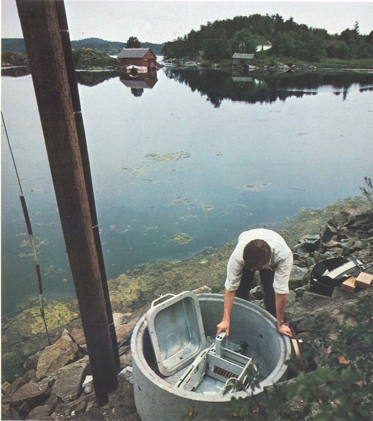
Ericsson's Pulse Code Modulation (PCM) system is used to boost line capacity between Arendal and Eydehavn in southern Norway. Photo shows one of the amplifiers used along the line.
