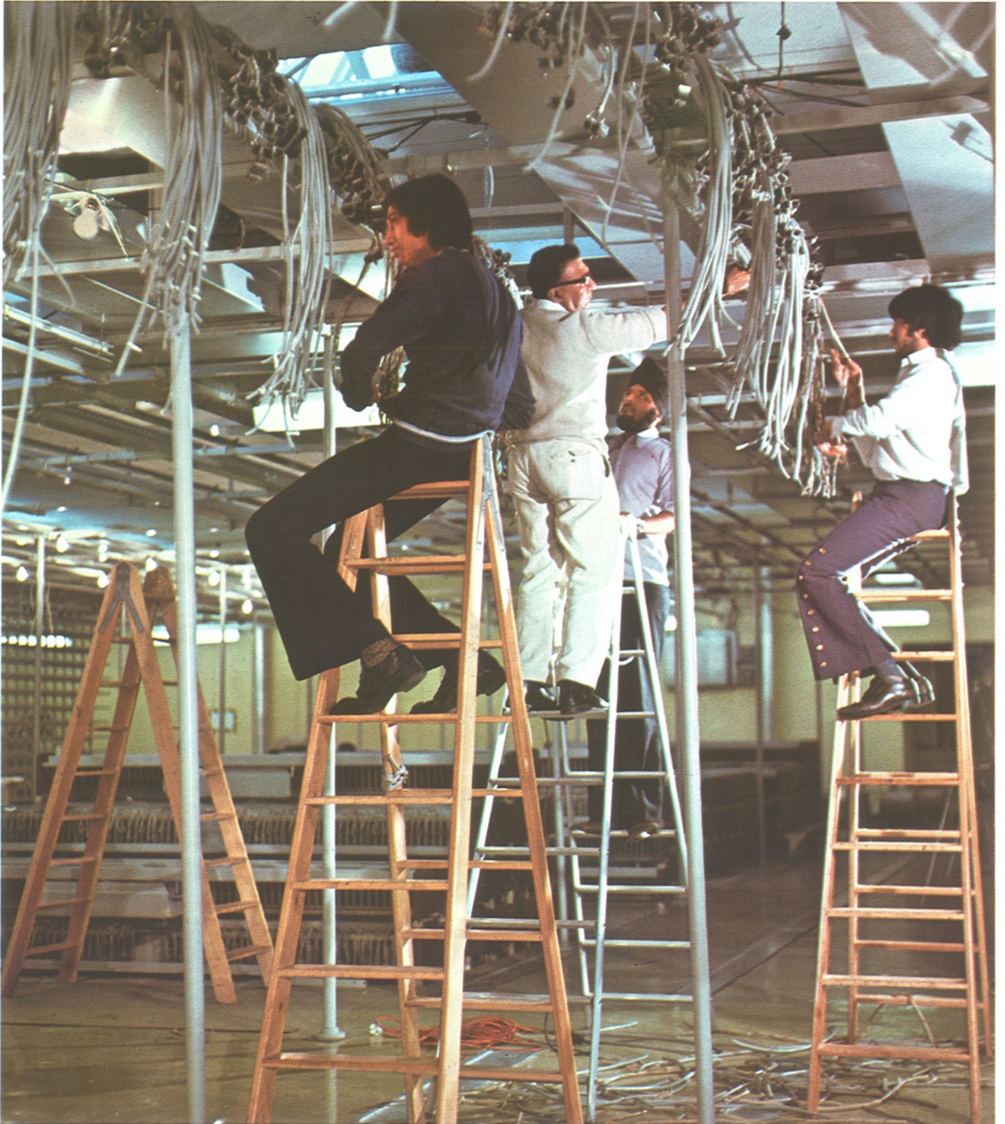
Installation of a telephone exchange for international traffic in Mollison House, London. The exchange, based on Ericsson's crossbar technique, is Ericsson's largest installation.
