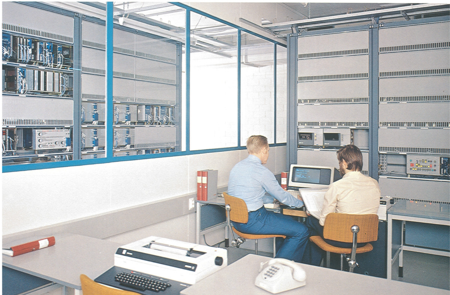
Control room in the new AXE telephone exchange in Turku, Finland, the first to be equipped with digital group selectors.
