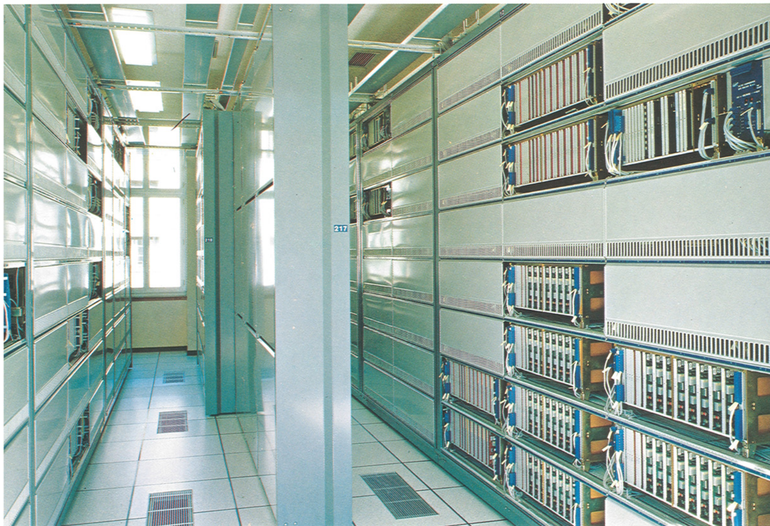
Interior of the AXE exchange in Orleans, France.
