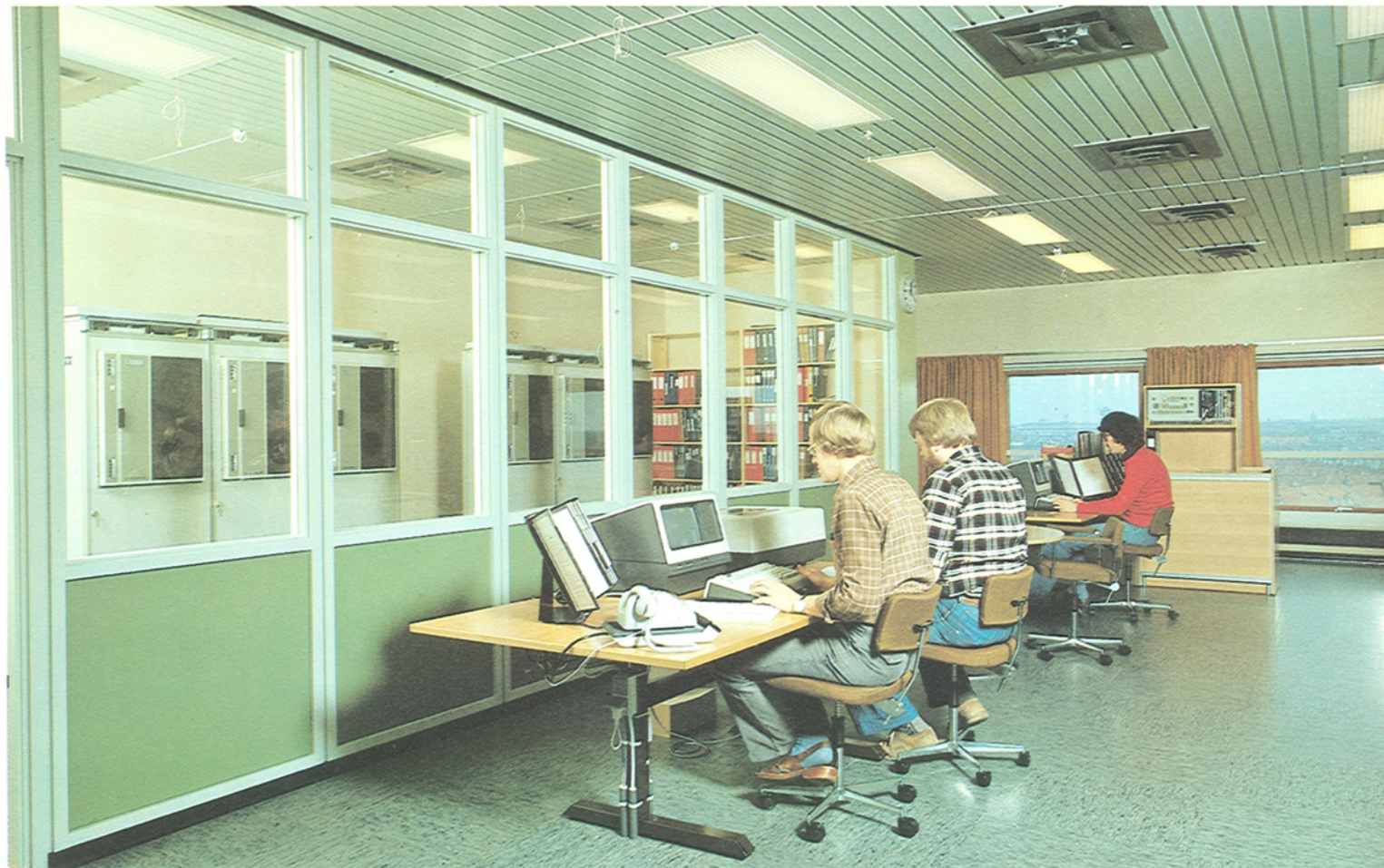
The first phase of the Nordic data network includes four AXB 30 computerized switching systems. This picture shows the control room in the Copenhagen exchange center.
