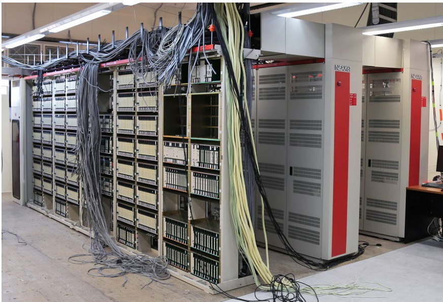
PSTN switches being decommissioned.
