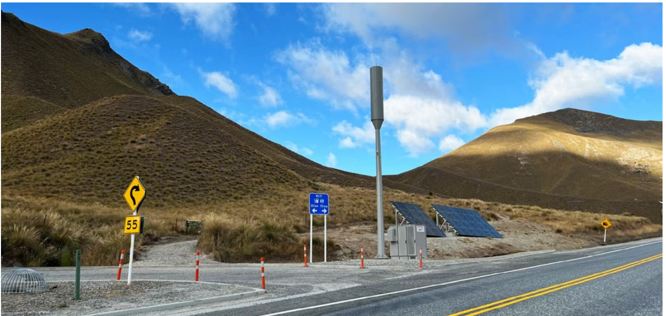
RCG cell tower at Lindis Pass providing mobile coverage for 4km of State Highway 73, powered by 36 solar panels.
