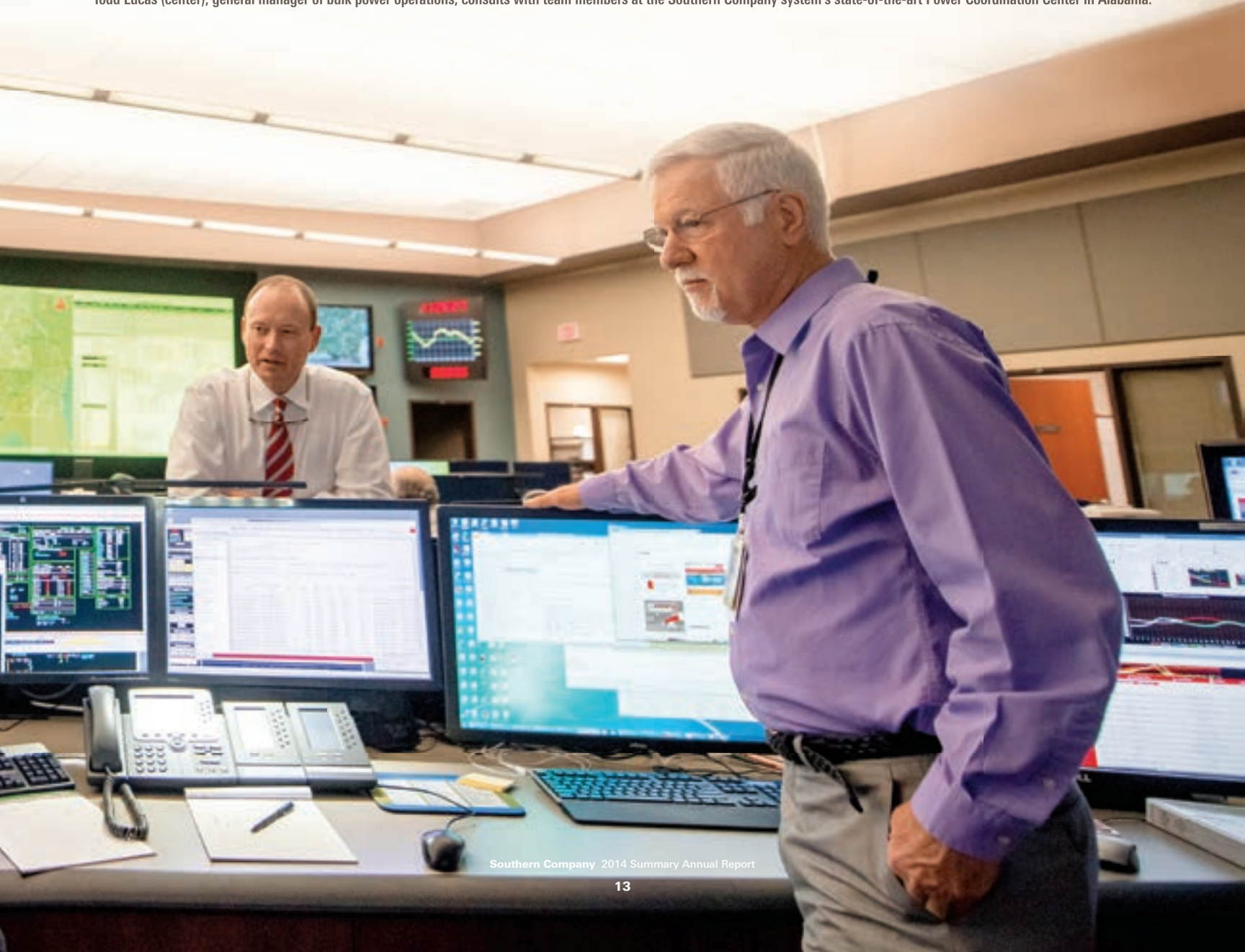
Todd Lucas (center), general manager of bulk power operations, consults with team members at the Southern Company system's state-of-the-art Power Coordination Center in Alabama.
