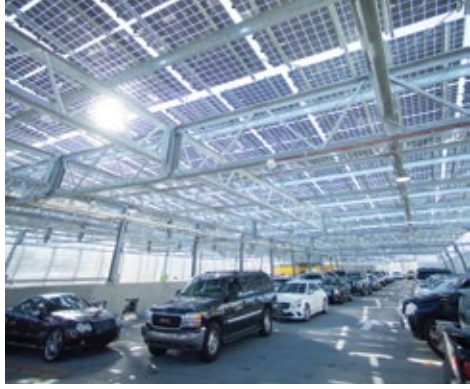
Georgia Power's solar installation at Mercedes-Benz Stadium helps the facility achieve its goal of 1.6 million kilowatt hours of energy per year from on-site solar generation.
