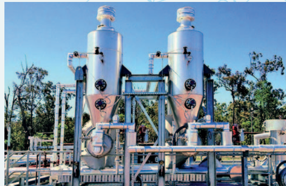
Typical Knock-out Pots used in ISG Demonstration Facilities (Source: Carbon Energy 2012 Annual Report).
