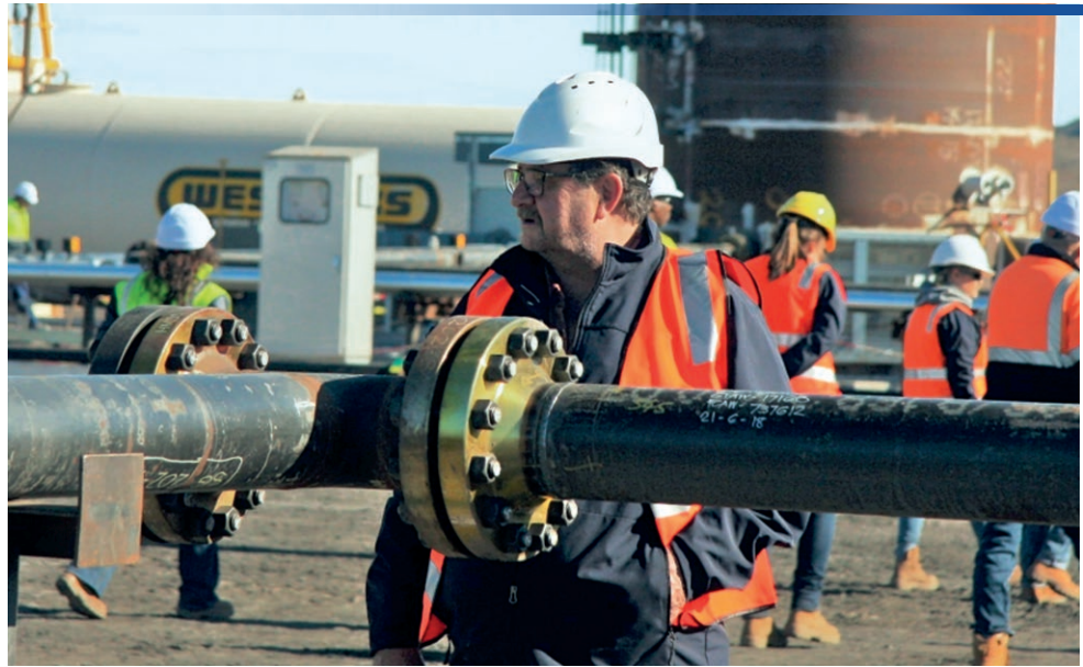
On site at Leigh Creek, Justyn Peters overlooking the construction of the demonstration plant.
