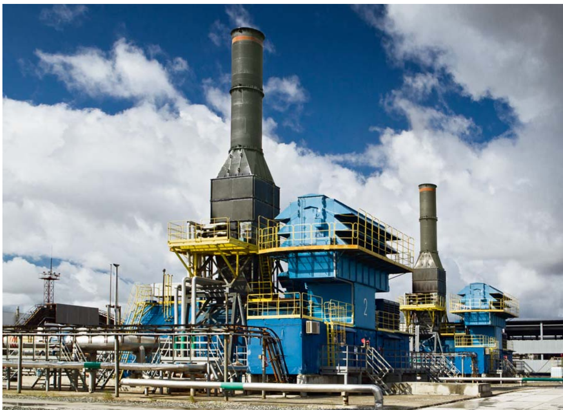
COMPRESSOR BOOSTER STATION AT THE EAST-TARKOSALINSKOYE FIELD
