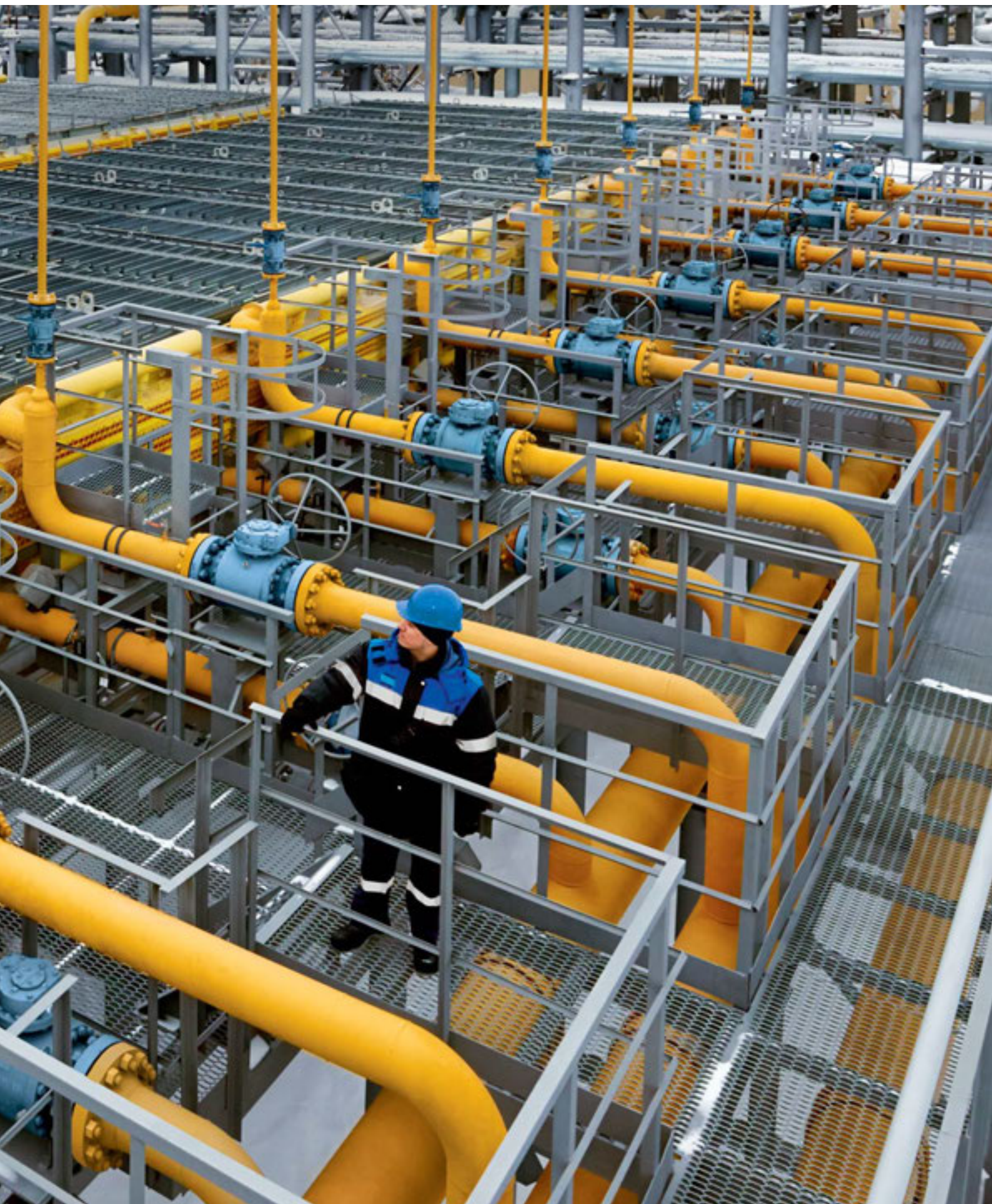
Yurkharovskoye field, compressor booster station. March 2014
