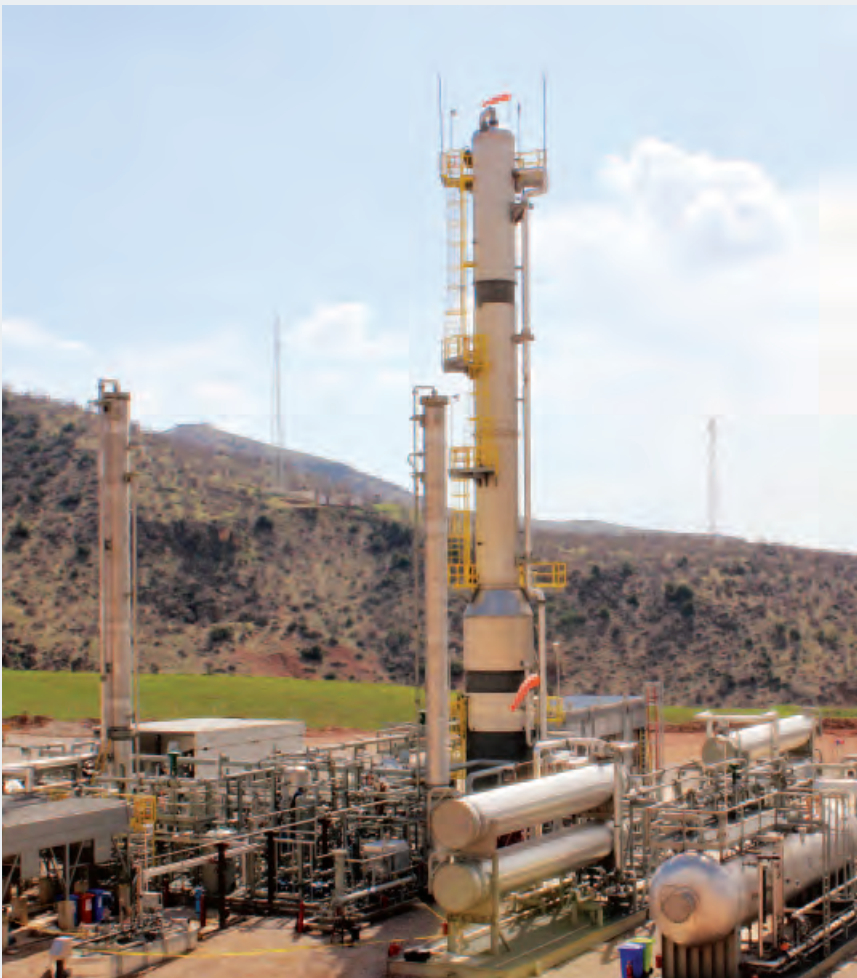
Shaikan production facility PF-1
