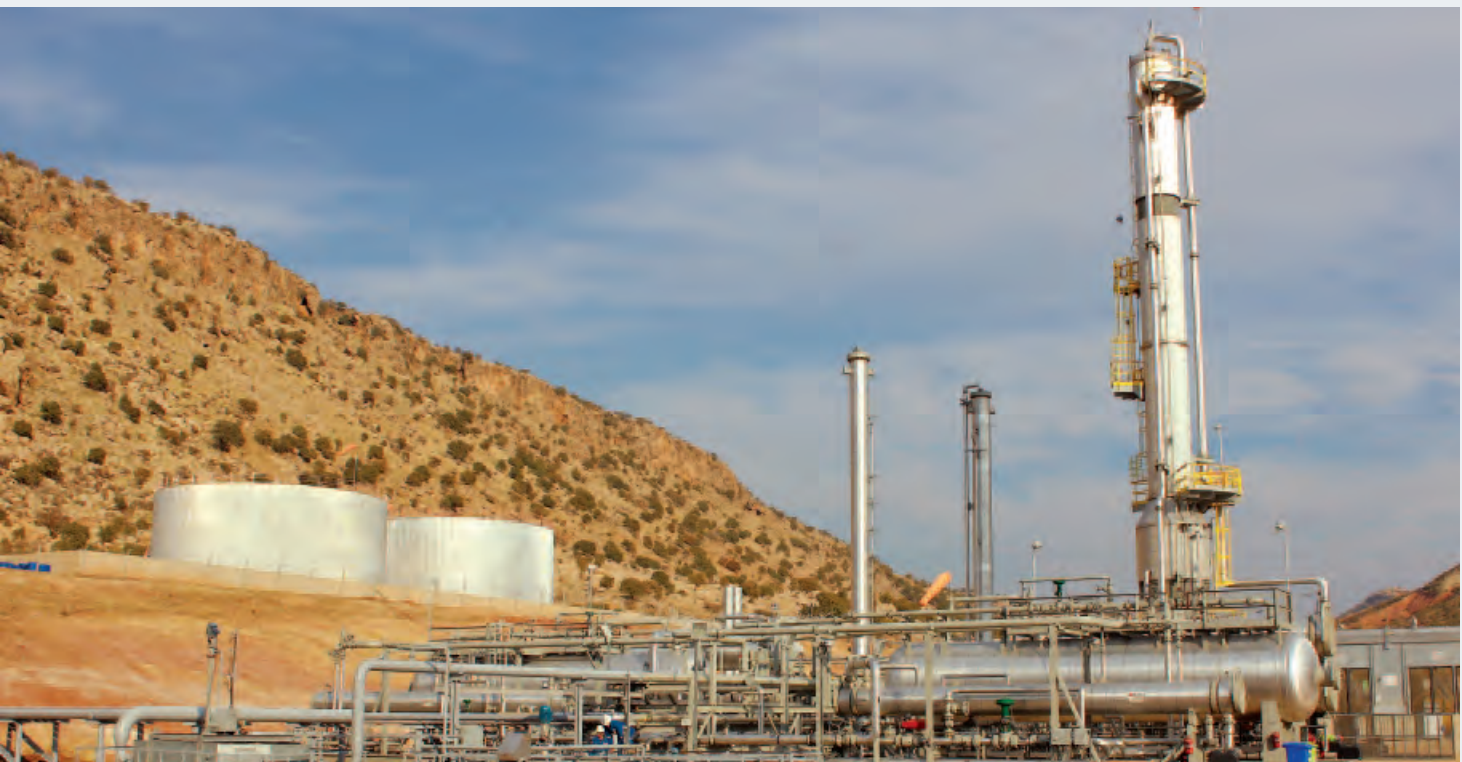
Shaikan production facility PF-1
