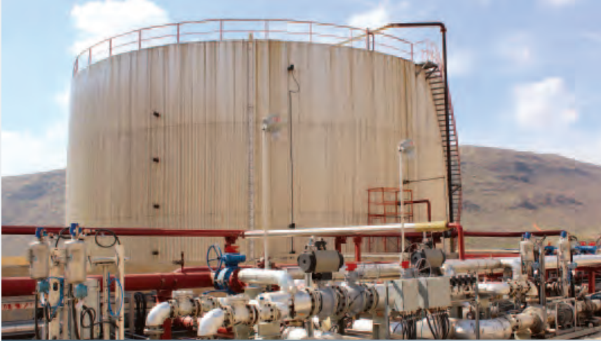
Storage tank at Shaikan PF-1
