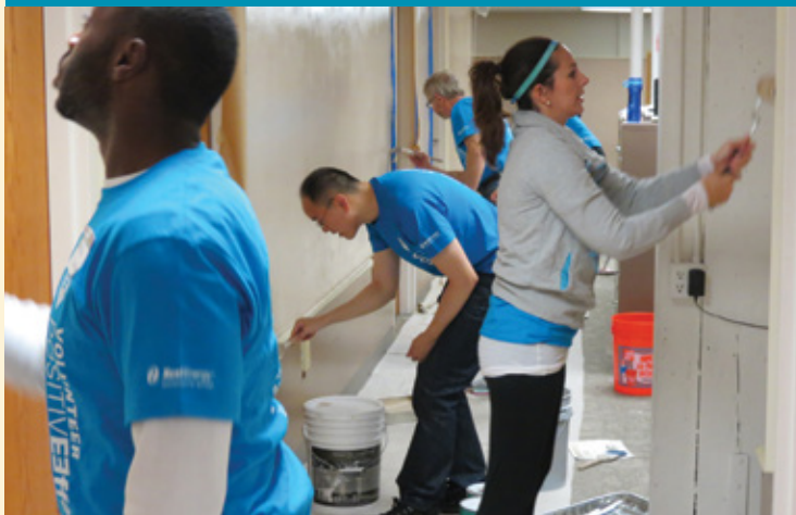
Xcel Energy volunteers Brandon Hassan, Alex Hassan, Roger Ly and Robert Hendricks (foreground to background) apply a fresh coat of paint during Xcel Energy's 5th annual Day of Service at AccessAbility, a Minneapolis non-profit that provides opportunities for self-sufficiency for people with barriers to employment and community inclusion.
