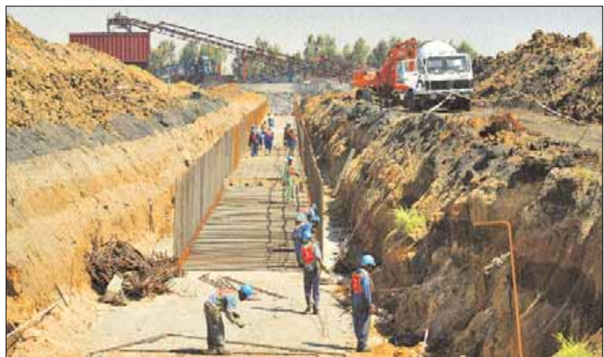
Construction of the Leeuwpán jig plant which will enable production of a further 1Mtpa of power station coal.
