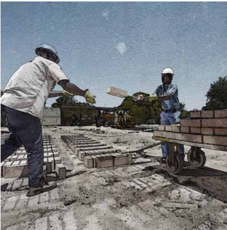
The rapid development in Lephallale increased demand for housing, in turn creating a business opportunity in the construction industry
