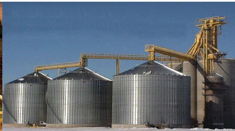
Hansen Installation: Fill Conveyors and Support Walkways
