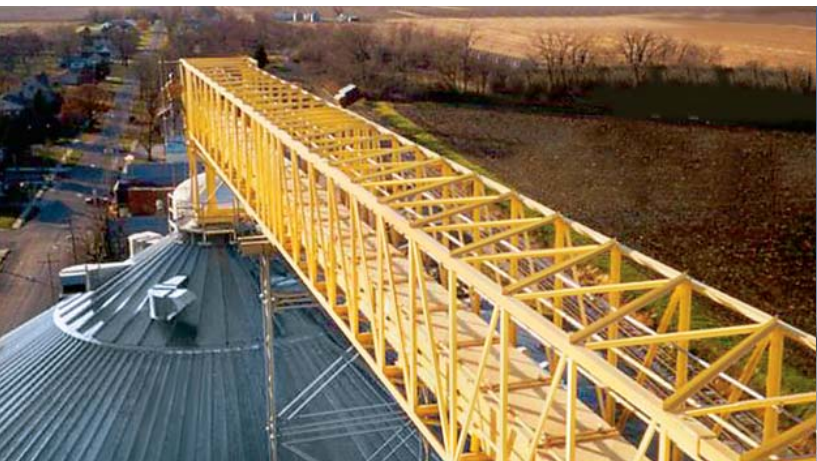
Hansen Installation: Conveyor and Support Walkway
