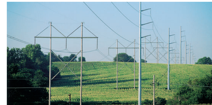
More and more utilities are finding it cost-effective to switch from wood poles to more reliable steel poles.
