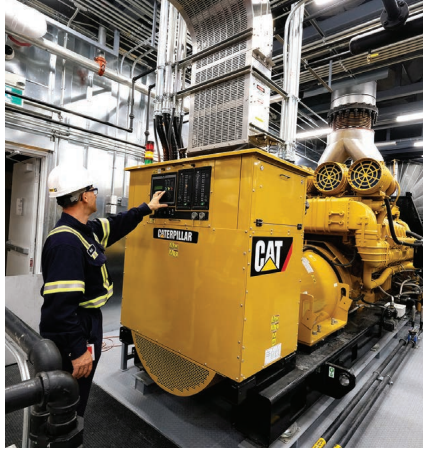
A Toromont technician inspects a Cat C-175 generator, which provides mission critical power for mining, data centre and hospital applications.
