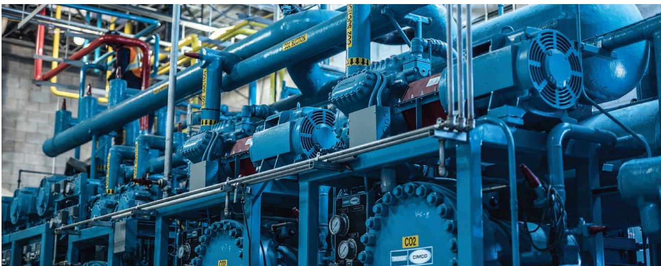
CIMCO designed this industrial-grade carbon dioxide/ammonia cascade system to provide superior performance using natural refrigerants.
