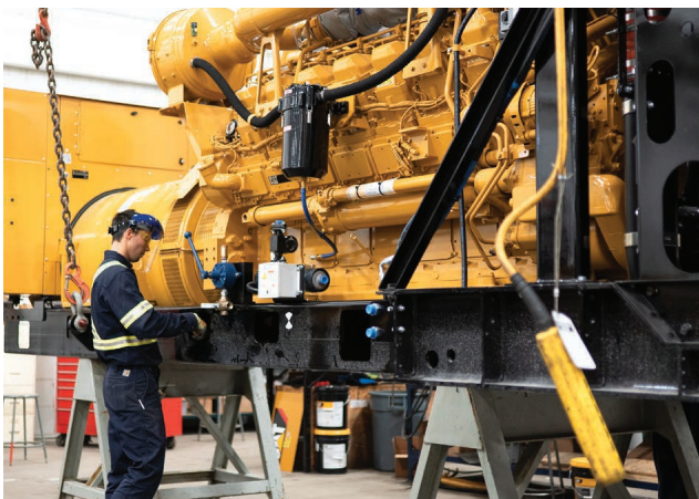
Toromont's Aaron Wright is part of a team at our Power Systems operation in Brampton, Ontario, that customized this Cat 3516 diesel generator for a customer's mission-critical application.
