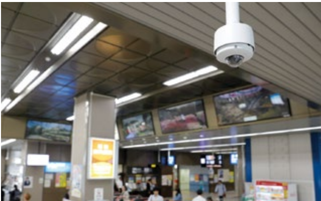
Network cameras at a Fukuoka City Subway station (Fukuoka, Japan)
