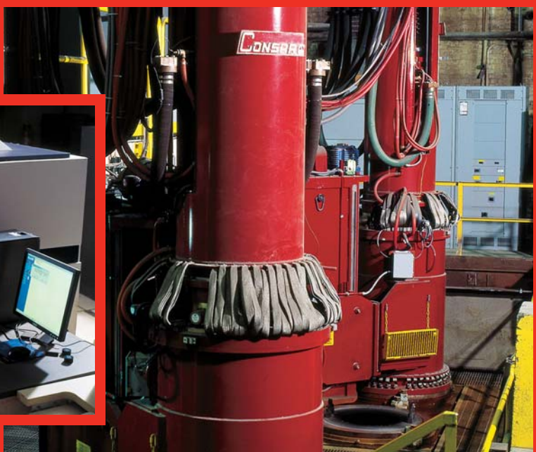
VAR Furnace / Bridgeville, PA
