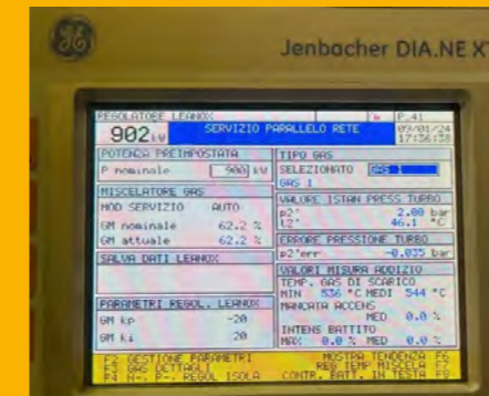
The gas engine meter indicates electricity production at 902kW, approaching the full capacity of the plant.
