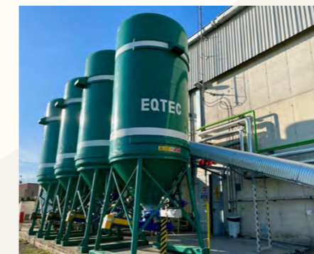
Four external hoppers capture approximately five days' worth of biochar output by the thermal cracking reactor inside the plant.
