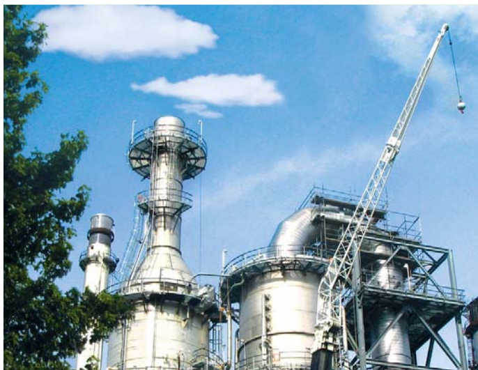
Valero's state-of-the-art scrubber units like this one at the Delaware City refinery reduce sulfur dioxide emissions by over 95 percent.
