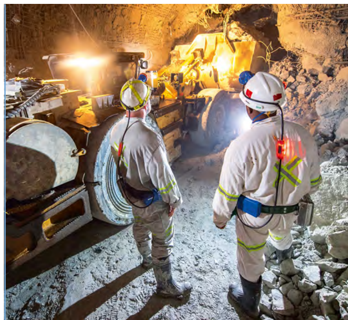
A Caterpillar LHD loading and cleaning an end during rehabilitation activities at Cullinan Mine.
