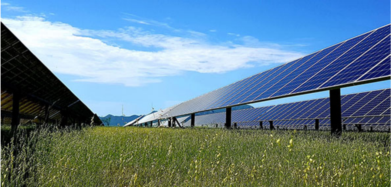
Hermsillo solar photovoltaic power plant - Sonora, Mexico
