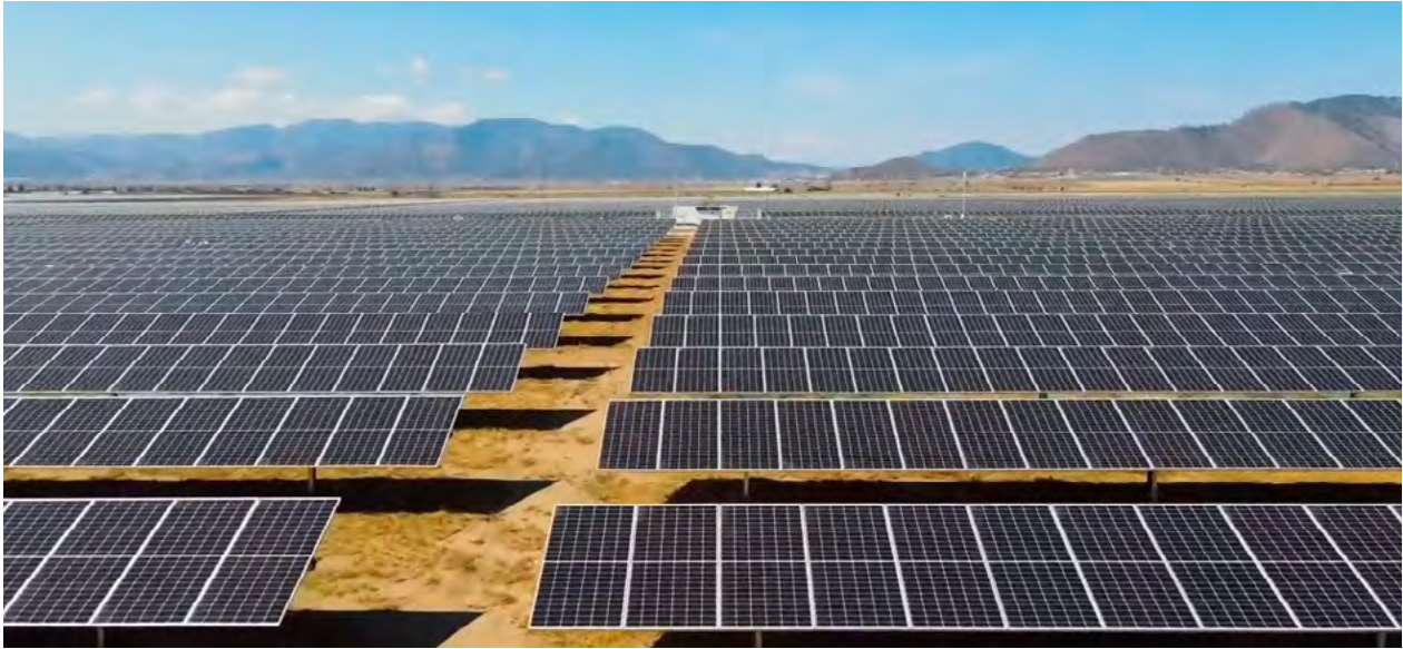
Cuyoaco solar photovoltaic power plant - Puebla, Mexico
