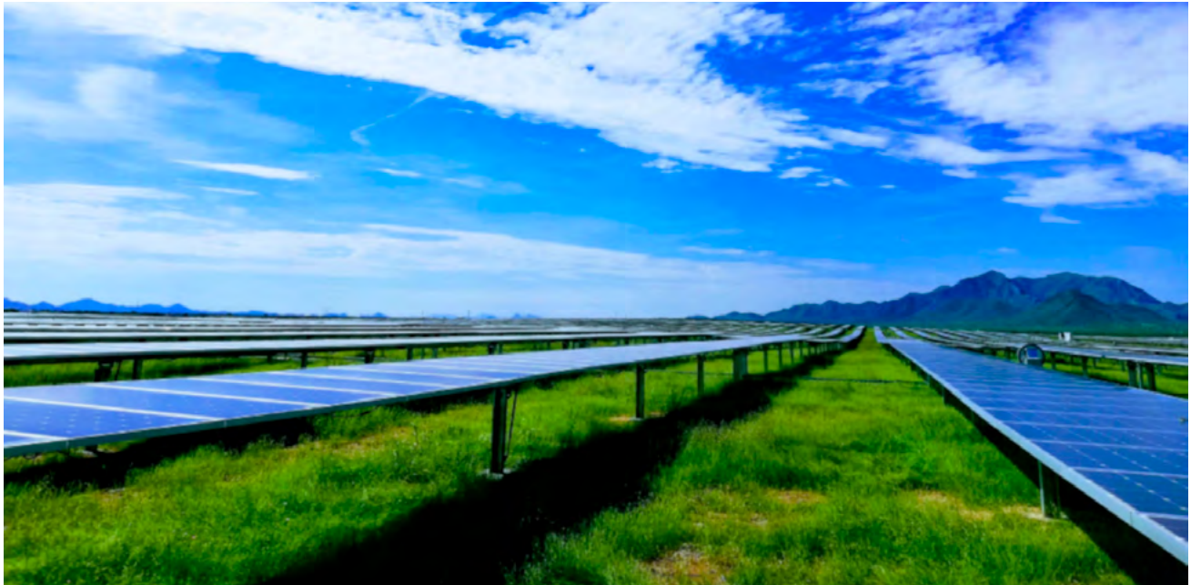
Hermosillo Solar photovoltaic plant, Sonora, Mexico
