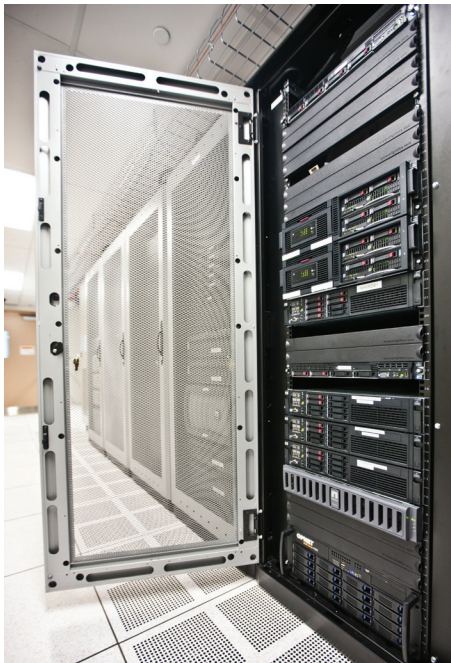
The new data centre at CWB Group’s corporate office stores more data in less space, which saves money and reduces our impact on the environment.
