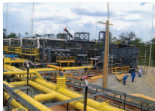
Contract compression units in Brazil
