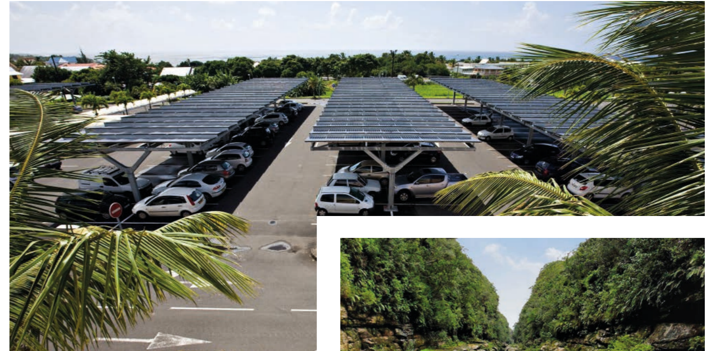
— Since 2007, the Casino Group has drawn on the expertise of its subsidiary GreenYellow to install 65 solar power generation units on roofs and solar canopies at car parks, and to operate 15 self-consumption systems.
