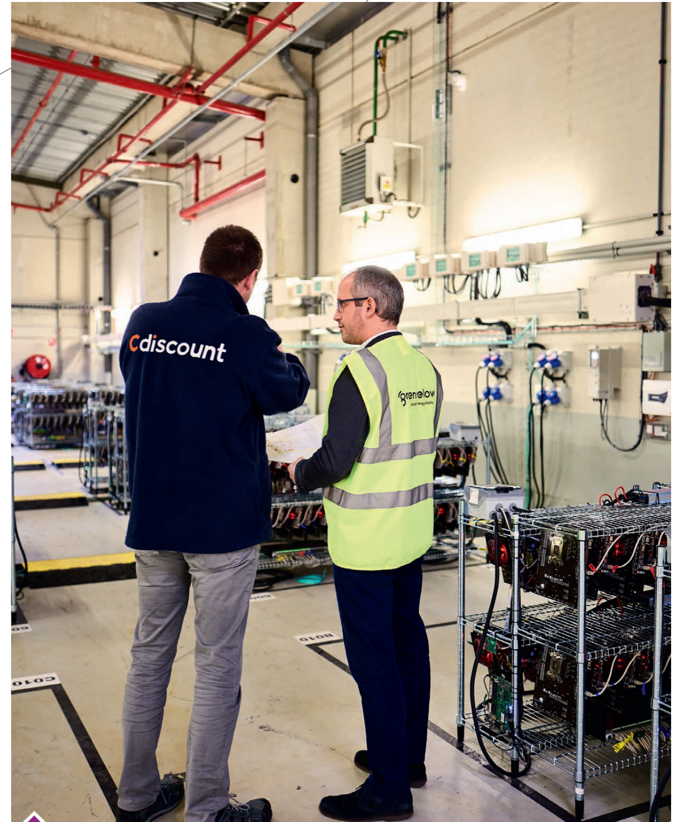
GreenYellow has installed a heat recuperation system in the ScaleMax Data Center located in Cdiscount's warehouse at Réau near Paris.
