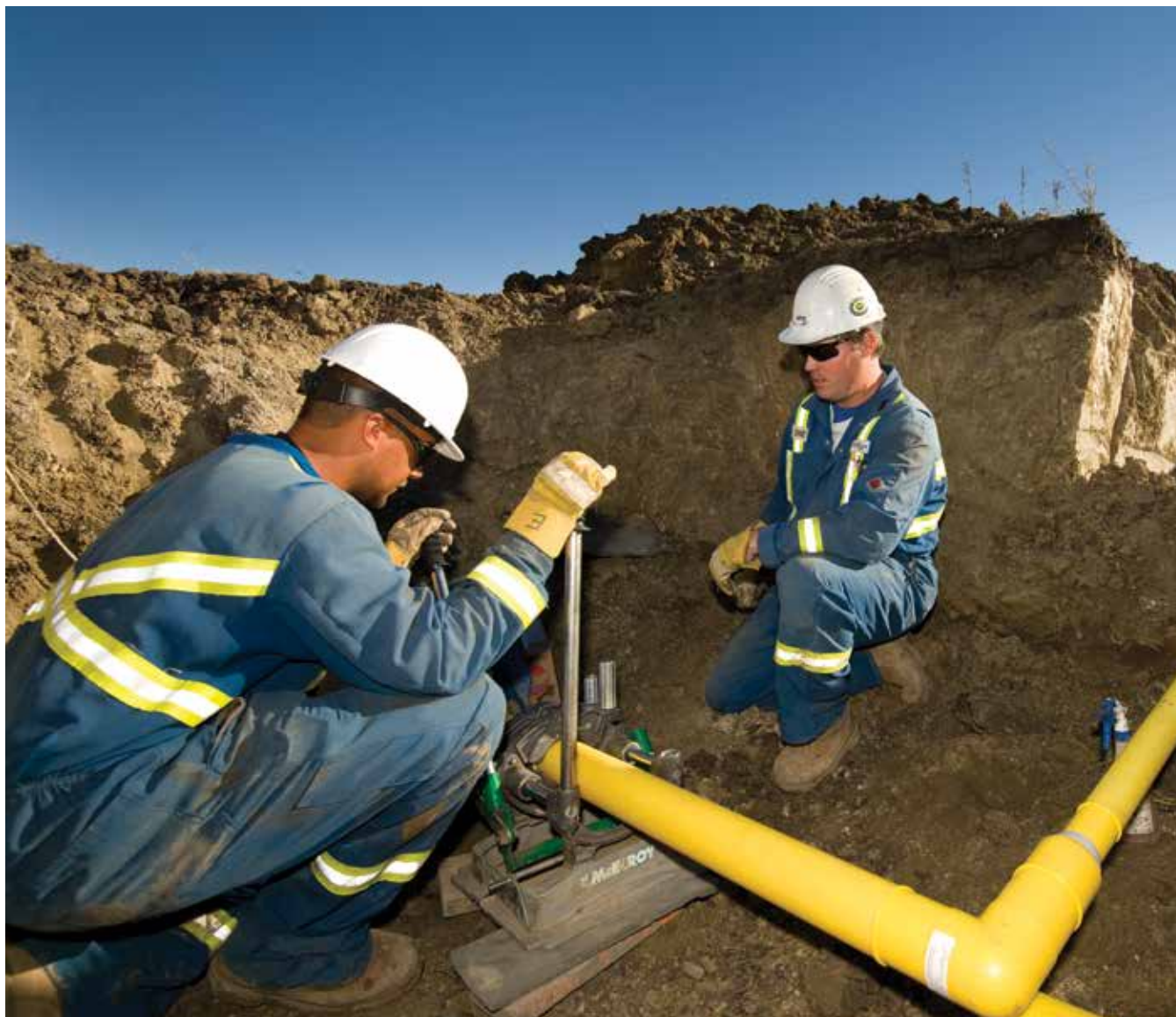
ATCO Gas Distribution Operators – Field, Evan Kostiuk (left) and Dave Swan, undertake a plastic mains replacement project east of Sherwood Park, AB.
