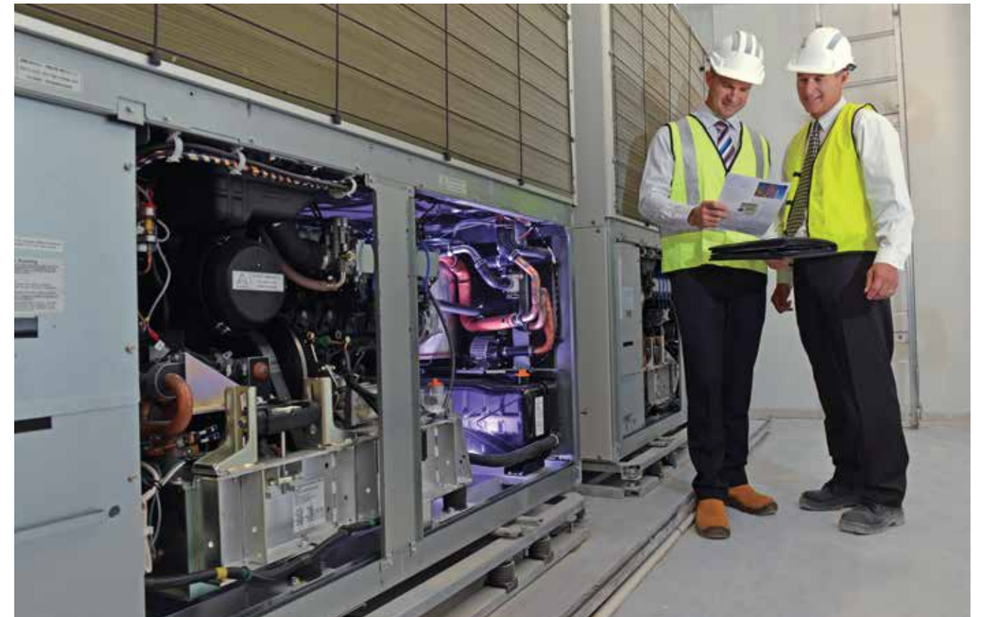
ATCO Gas Australia's President, Alan Dixon, and Business Development Manager, Nathan Lude, inspect the natural gas-fired air conditioning system recently installed at the company's Jandakot building.
