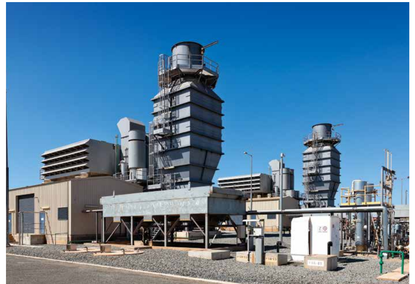
The home of ATCO's 86 MW Karratha Power Station in the resource-rich Pilbara in northwest, Western Australia continues to be a focus for ATCO Australia.
