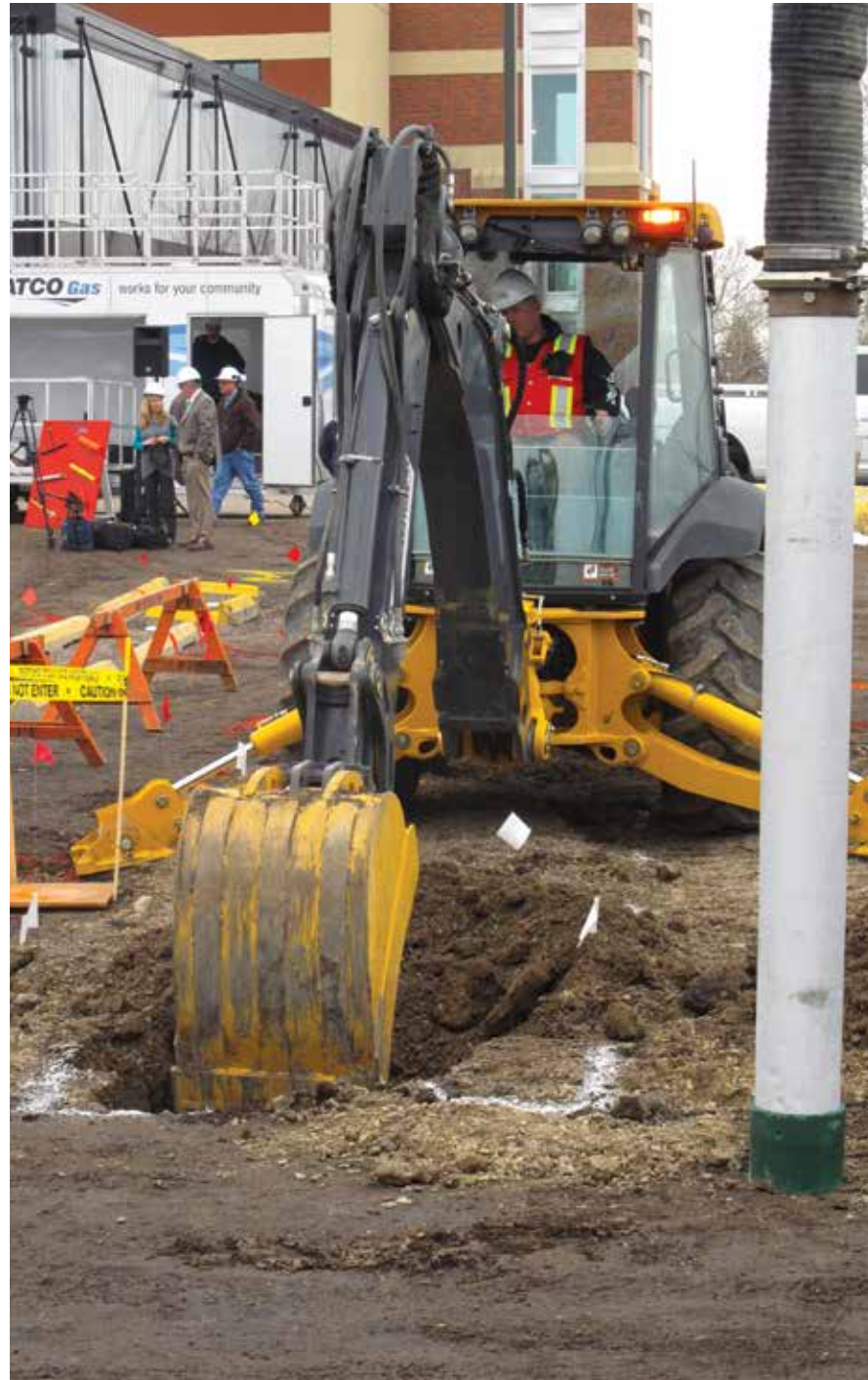
In support of Safe Digging Month, ATCO Gas led the Alberta Common Ground Alliance's live excavation demonstration at the Southern Alberta Institute of Technology.
