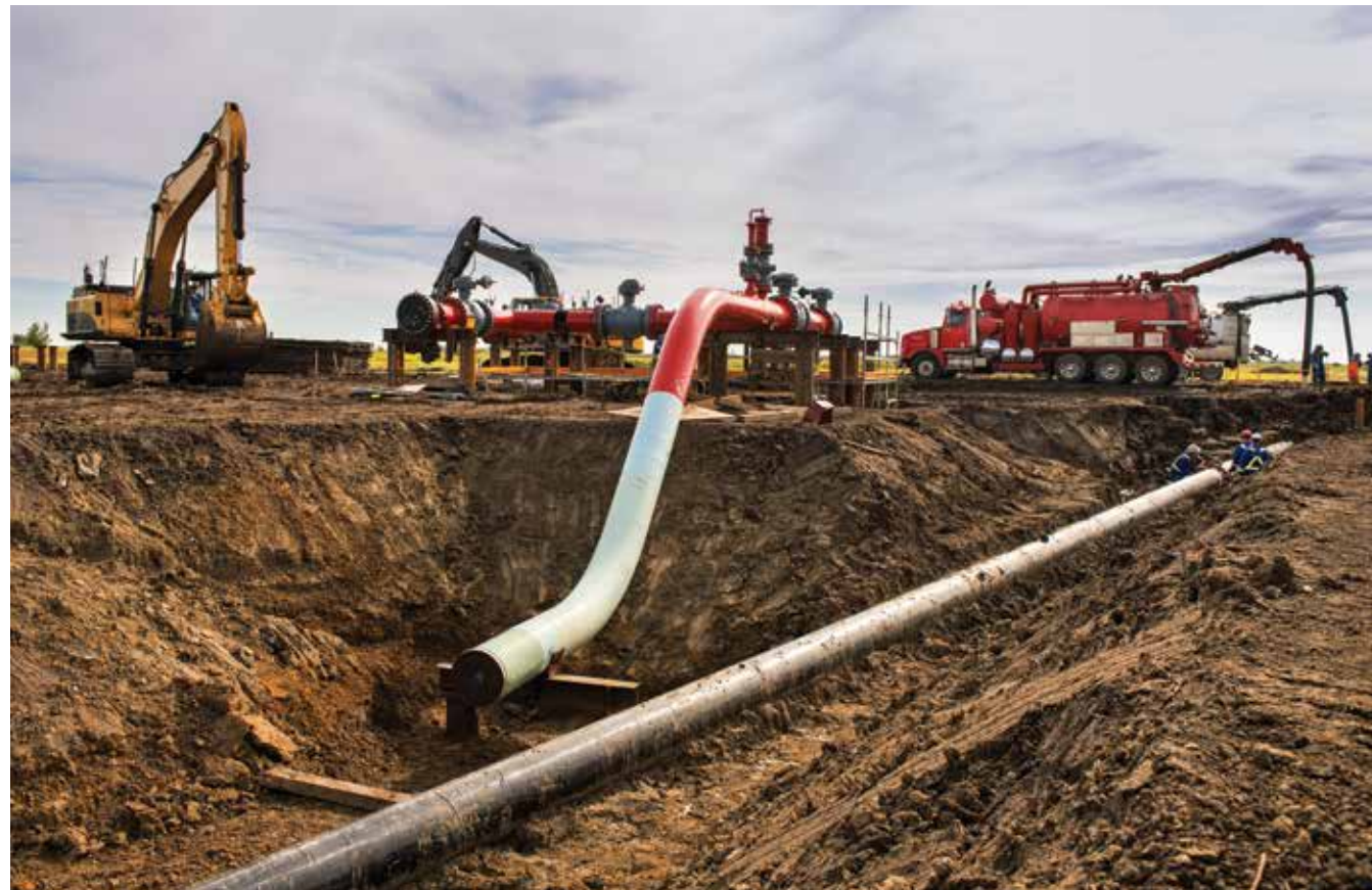
Construction crews installed 41 km of 508 mm (20 inch) pipeline in Norma, AB, to ensure sufficient supply of natural gas to meet growing demand in the Fort Saskatchewan and Edmonton regions.
