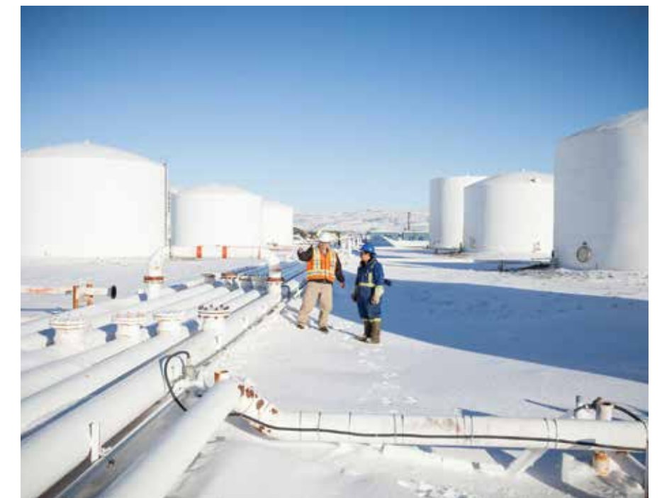
UQSUQ Corporation, a joint venture between Nunavut Petroleum Corporation (representing the Nunasi Corporation and Qikiqtaaluk Corporation) and ATCO Structures & Logistics, operates the 79 million litre bulk fuel storage facility in Iqaluit. The facility meets the refueling needs of Iqaluit airport and supplies the City of Iqaluit with fuel.
