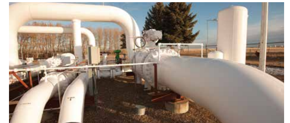
ABOVE: The Empress Gas Liquids Straddle Plant processes up to 1.1 billion cubic feet/day.
