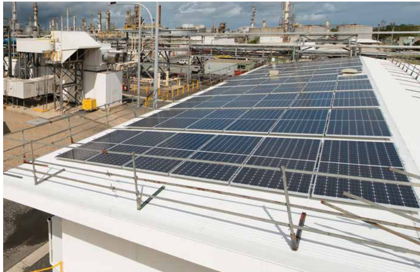
Solar panels installed at the Bulwer Island facility are part of a focus of ATCO Power Australia to improve the energy efficiency at all of its facilities.
