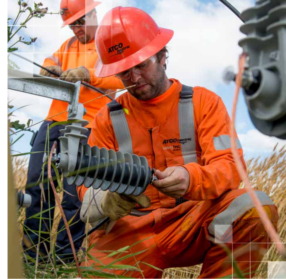
Dallas Fjeld, Equipment Operator (back) and Brad Gerbrandt, Powerline Technician - Line (front), replace a gang switch near Grande Prairie. ATCO's electrical system serves more than 224,000 customers in northern and east-central Alberta.
