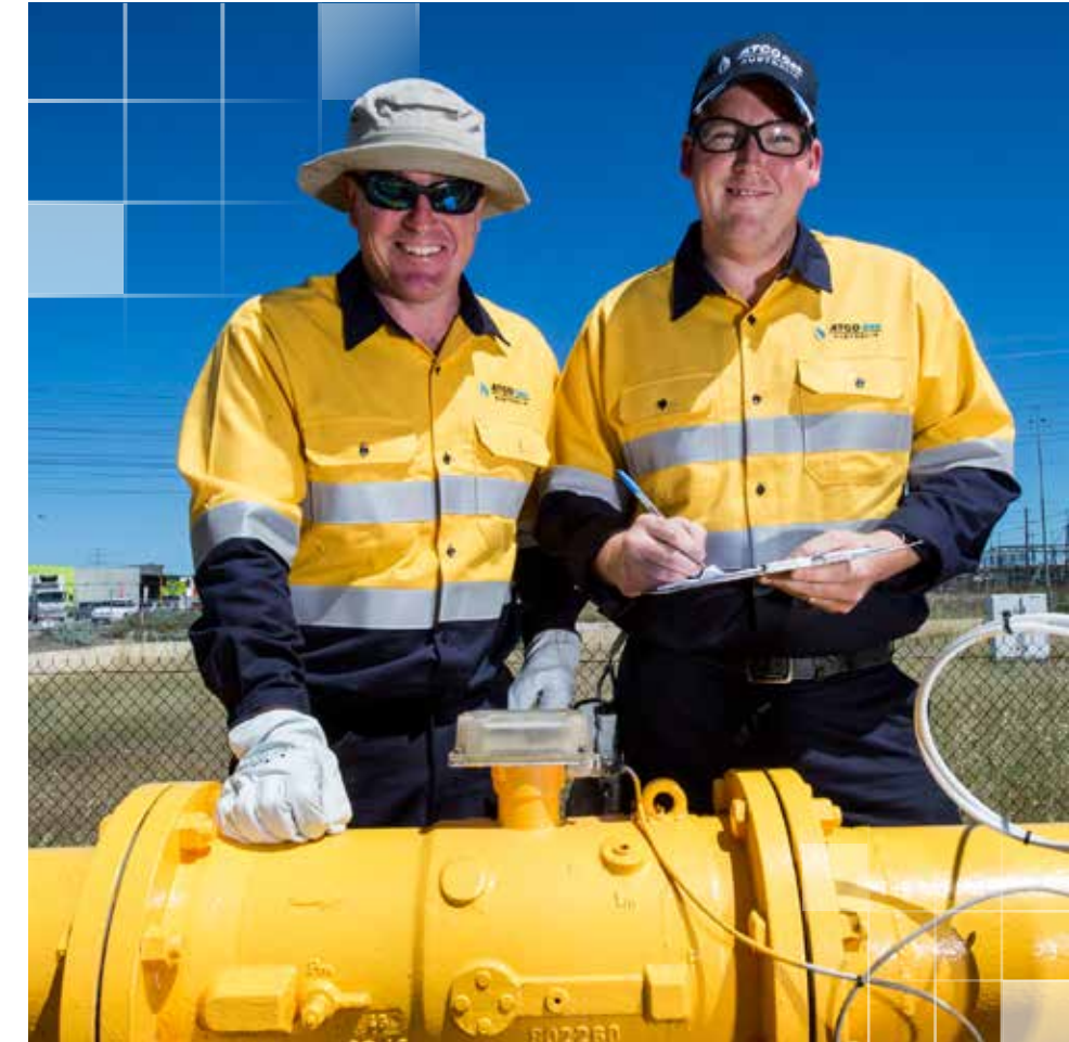
Jody McNeill and Pete Dainton, Gas Distribution Officers, Facilities Maintenance at ATCO Gas Australia, service the pressure reduction station in Ballajura to ensure the safe and reliable delivery of natural gas for consumers in Perth and surrounding regions.
