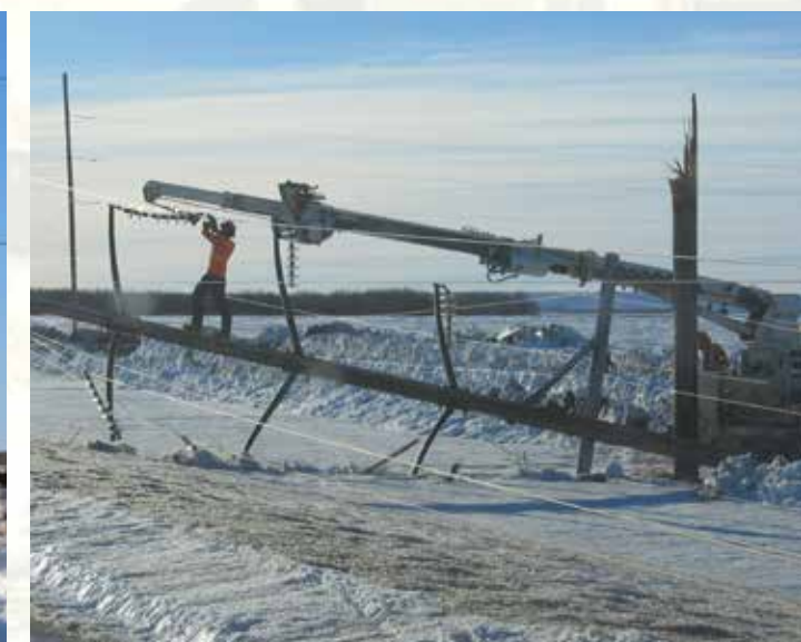
Dangerous public hazards like the toppled transmission structure shown here characterized the damage caused by the windstorm. ATCO Electric crews responded immediately, restoring power to more than 85 per cent of its customers within the first 36 hours.
