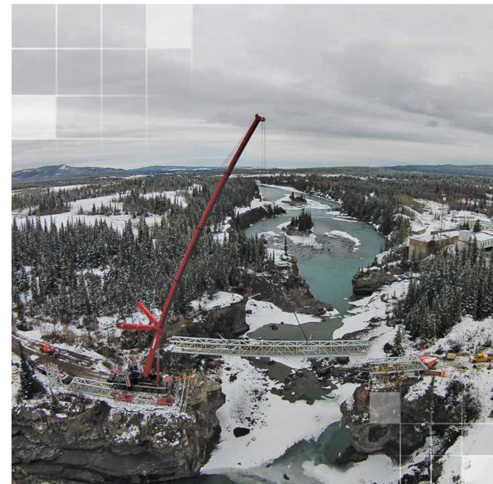
ATCO Pipelines successfully completed a new aerial crossing along the Banff Transmission Pipeline, near Seebe, Alberta. Originally installed in 1951, the pipeline was suspended from a vehicle bridge no longer fit to safely support the pipeline river crossing.
