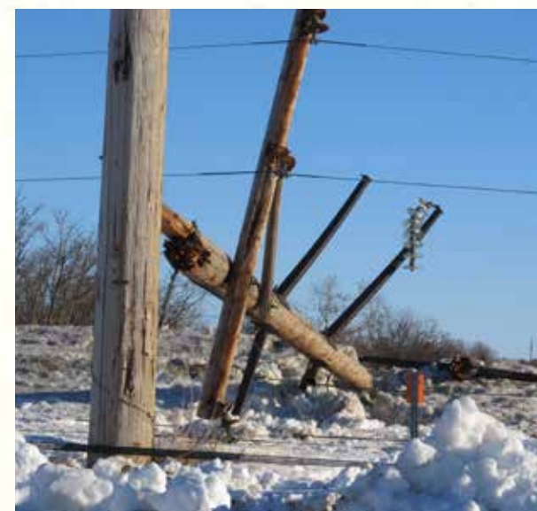
In January, severe windstorms resulted in extensive damage to transmission towers and distribution poles throughout northern Alberta, leaving more than 14,000 ATCO Electric customers without power.
