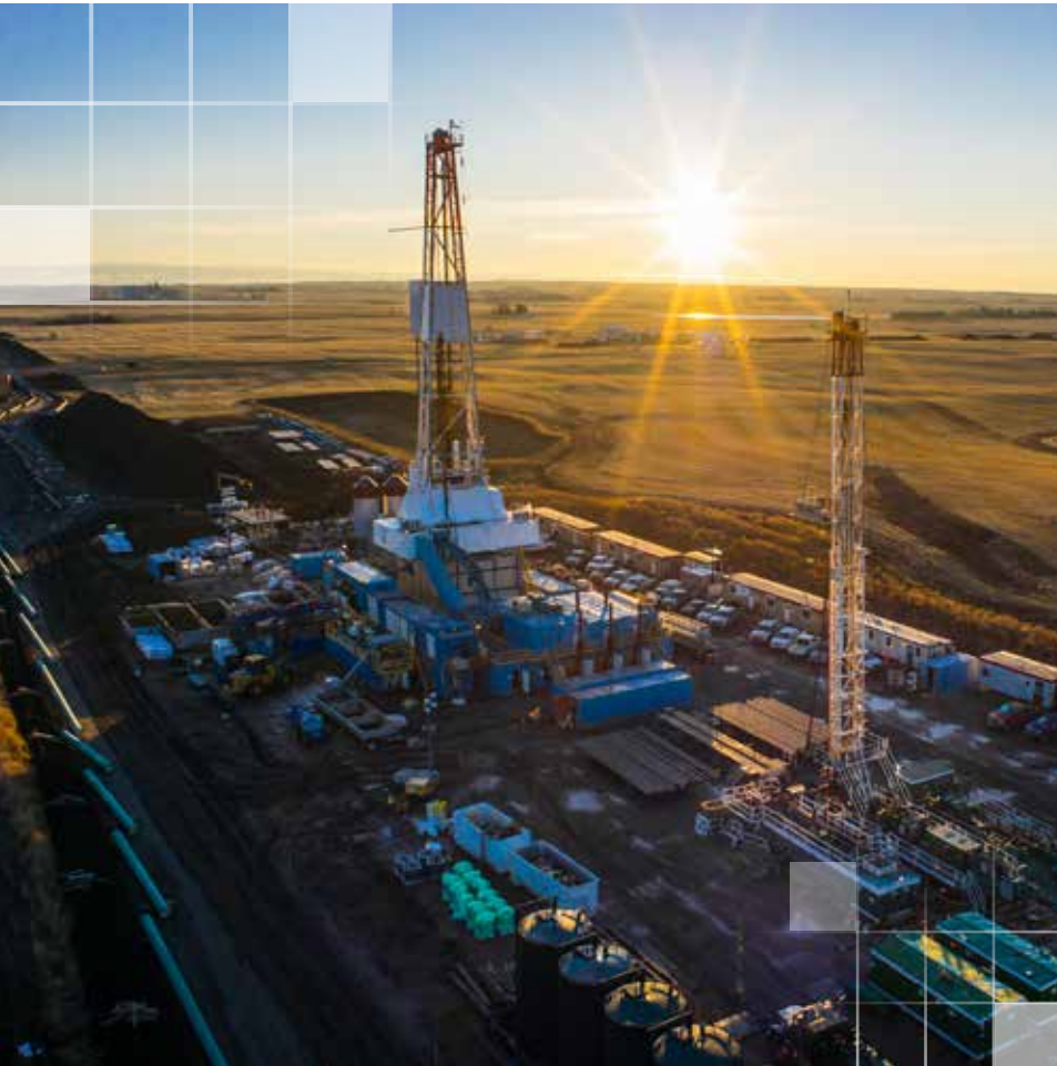
ATCO Energy Solutions recently doubled its land position in Alberta's Industrial Heartland, an area critical to Alberta's energy industry. With the additional 160 acres of land, the company has the potential to develop more than 40 salt caverns on ATCO-owned land in the area.
