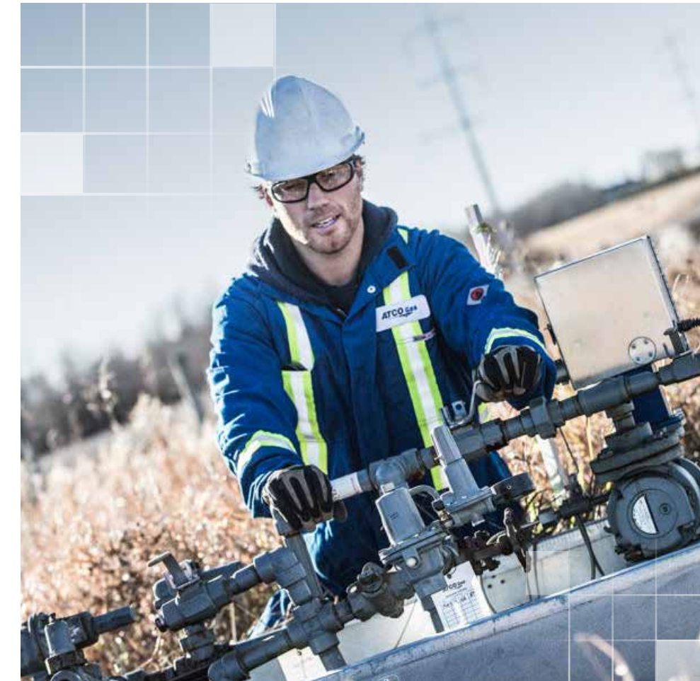
As part of a large distribution system upgrade, ATCO Gas employee Brad Trautman, Distribution Operator – Field, Camrose, works on a “farm tap unit” near Camrose, Alberta.
