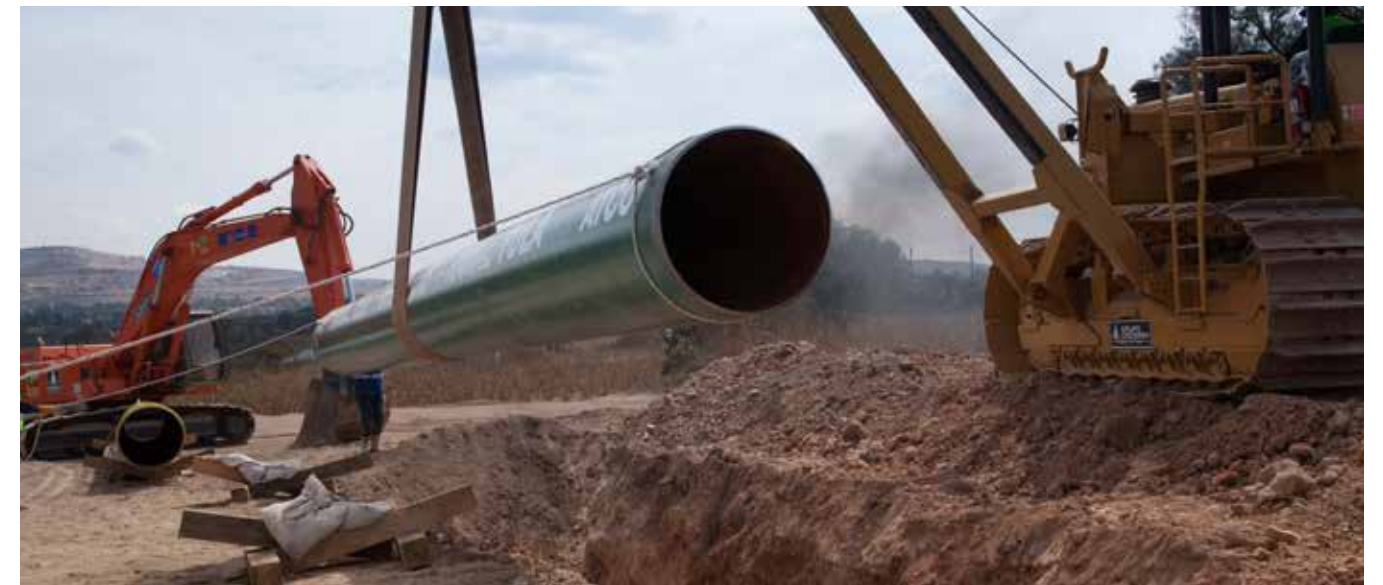
Construction of the Ramal Tula Pipeline Project in Mexico was officially launched in February 2015. Above, the first section of pipe is lowered into the ground.
