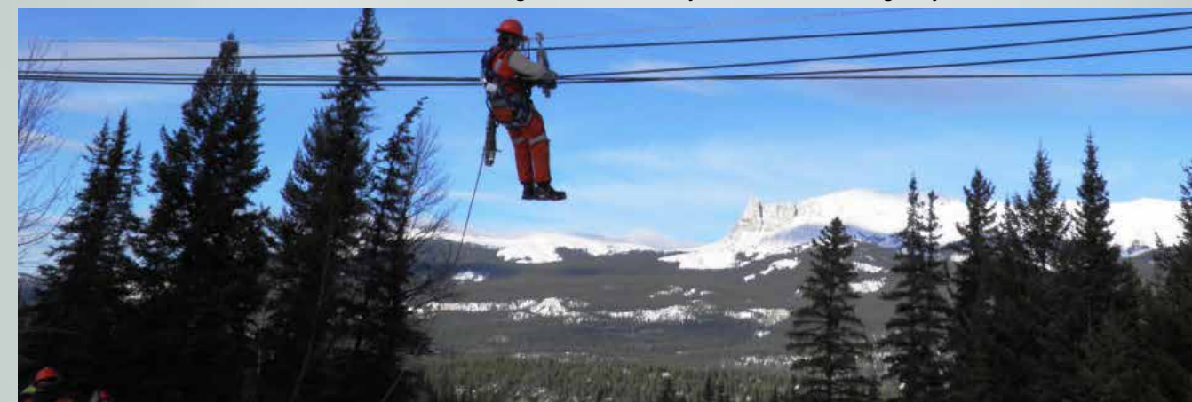
During the project, boatswain chairs were brought in allowing ATCO Electric crews to perform aerial work in areas not accessible by bucket truck.
