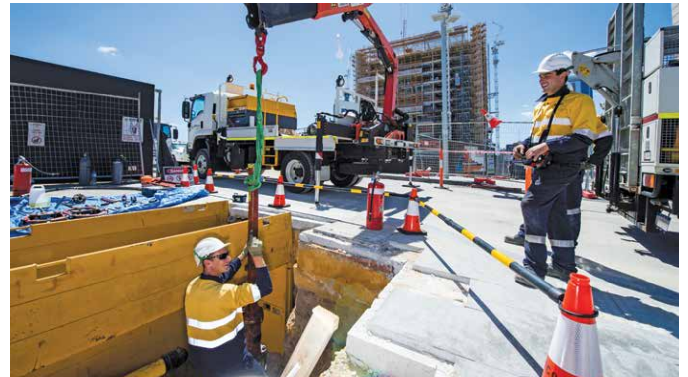
Nick Smith and Aden Bourke, Gas Distribution Officers, commissioning a new gas main pipeline to Kings Square in the Perth city centre, part of one of Australia's most significant urban renewal developments.
