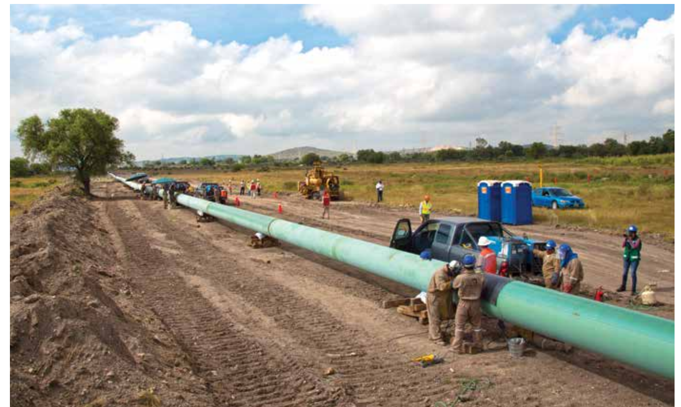
Construction on ATCO's Ramal Tula Gas Pipeline is well underway. The pipeline will transport natural gas to the Comisión Federal de Electricidad's Francisco Pérez Ríos thermoelectric power plant.
