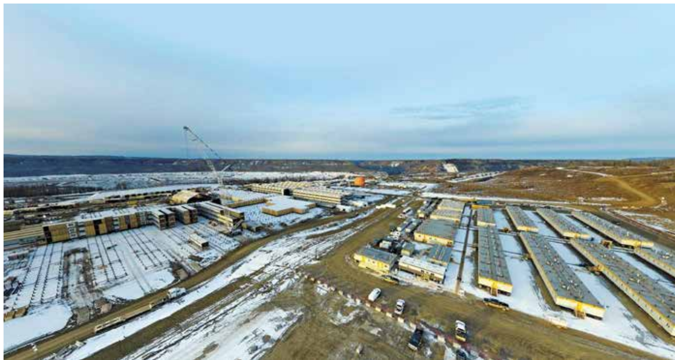
ATCO Structures & Logistics is building a temporary community in the form of a 1,600-person workforce housing facility for the construction of BC Hydro's Site C Clean Energy Project.
