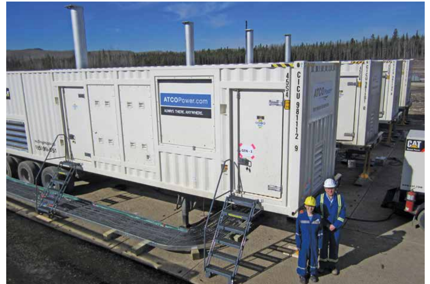
ATCO Power's Distributed Generation team successfully delivered a 5 MW temporary power generation solution that reduces flare gas for Apache Canada Limited. Temporary power solutions can be used to bridge the gap between grid connection and permanent generation for emergency or supplementary onsite power or to offset electricity shortages.
