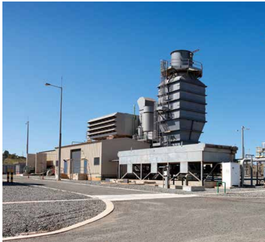
ATCO's Karratha Power Station is the most efficient and environmentally friendly facility in Australia's North West Interconnected System.
