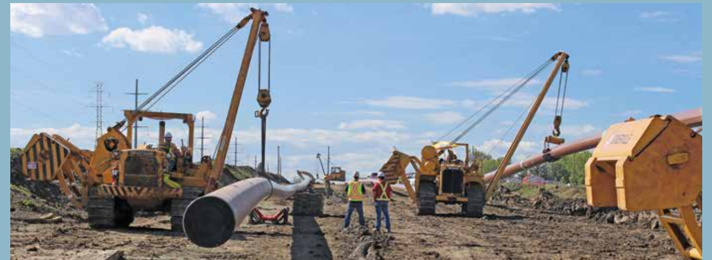
Through the UPR Program, ATCO Pipelines is building new, high pressure pipelines in Transportation/Utility Corridors in Calgary and Edmonton.
