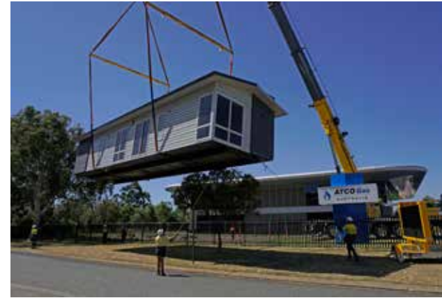
Our modular home being installed at the Clean Energy Hub in Australia is outfitted with the latest in cutting-edge energy technologies and showcases the integrated, customer-centric solutions we can deliver for customers around the world.
