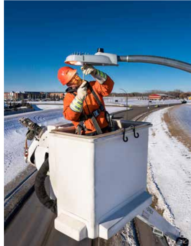
In Lloydminster, we converted outdated street lights to LED bulbs and installed intelligent street lighting sensors. The combined technologies reduce costs, maintenance
