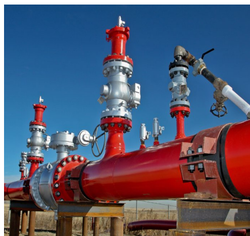
Natural Gas Pipeline Valve Assembly
