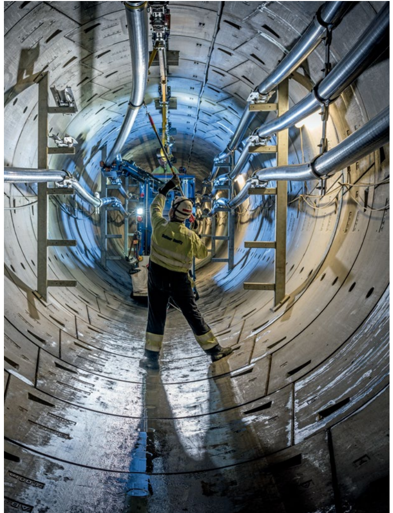
We’re installing high-voltage electricity cables in deep underground tunnels, protecting London’s future demand for energy.
