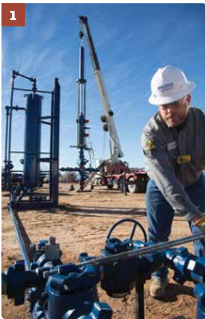
1 Wellhead isolation and flowback equipment and personnel supporting our customers in the Permian Basin.
