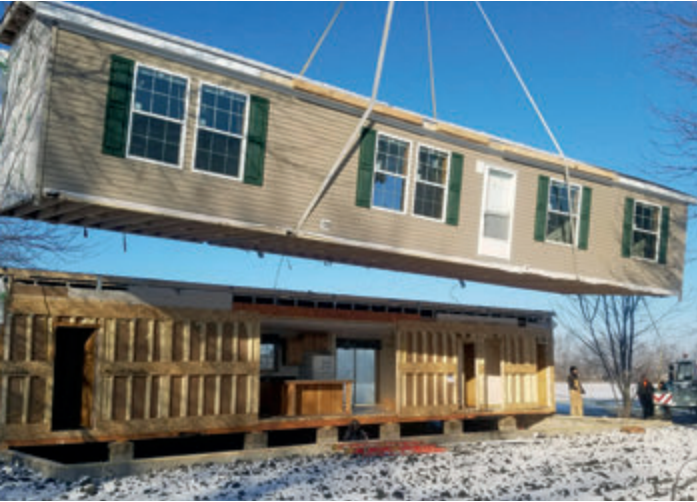
Modular Home Installation on Private Land by UMH Sales Center, Anderson, IN
