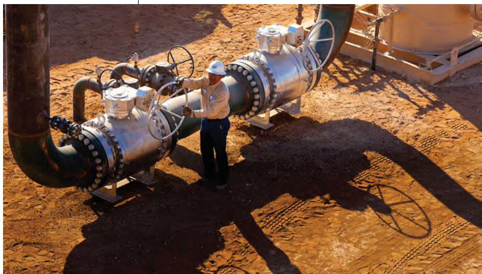
(ABOVE) Compressor station in the Eagle Ford shale, Dimmit County, Texas.
