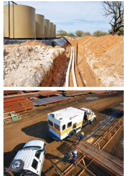
Top: A Flexpipe Systems installation in the oil-rich Eagle Ford shale formation in southern Texas.
