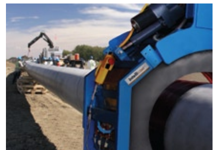
Top: Shaw Pipeline Services' proven HDUT technology provides state-of-the-art mechanized ultrasonic testing technology for the complete inspection of pipeline girth-welds.
