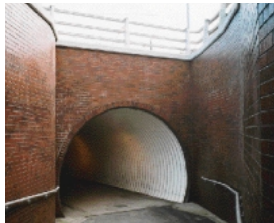
Pedestrian underpass in Carmarthen connecting residential area with superstore. Multiplate supplied by Asset with anti-graffiti paint system.
