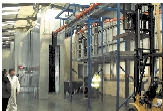
New powder coat plant at Barkers Engineering.
