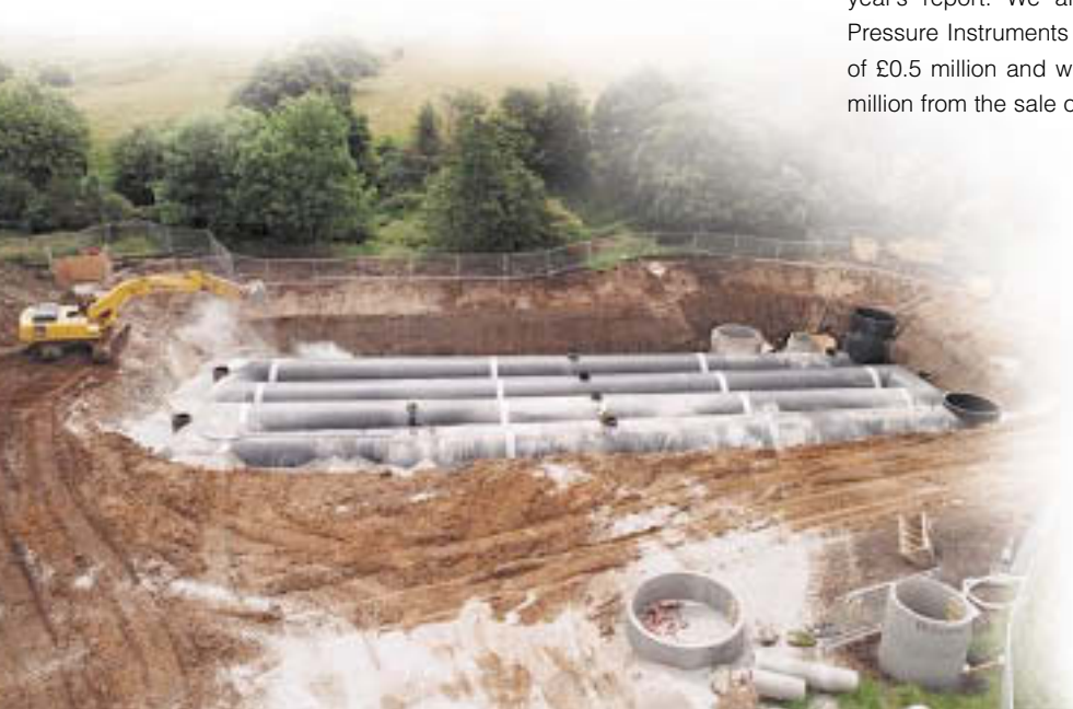
Combined sewer and storm water overflow tank, Bradford. AMP3 project for Yorkshire Water.
