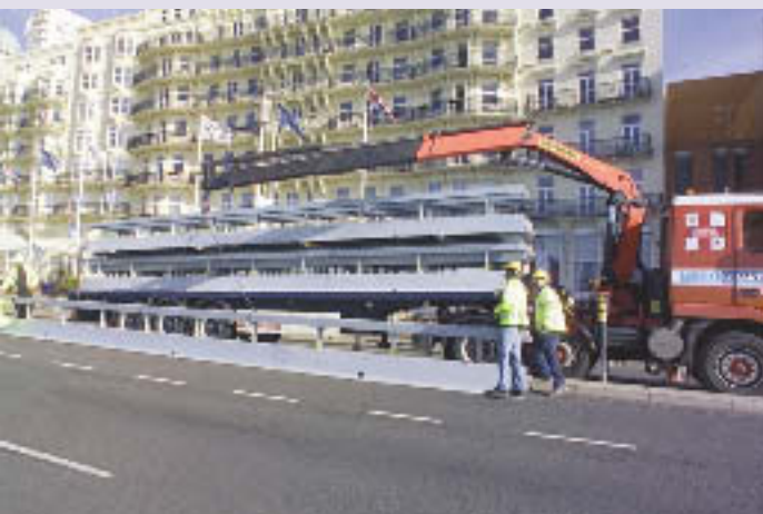
Asset International's steel safety barrier, "VARIOGUARD®", being installed at the front of the Brighton Centre in readiness for the Labour Party Conference.
