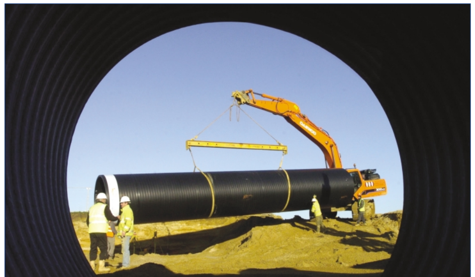
Right: A view through Asset International's "Weholite" drainage product showing installation at the new Arbury Park project, Cambridgeshire.
